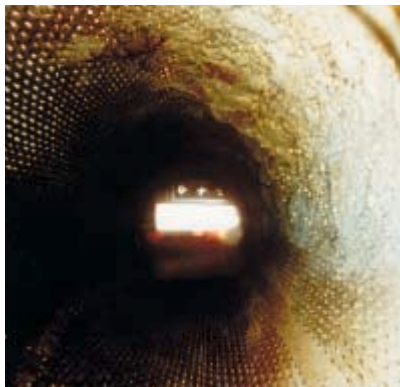
Well cleaning with high-pressure water right: prior to cleaning left and bottom: after cleaning
