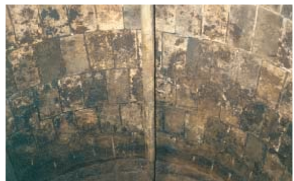
Incrustation removal from a stirrer upper: prior to cleaning, lower: after cleaning
